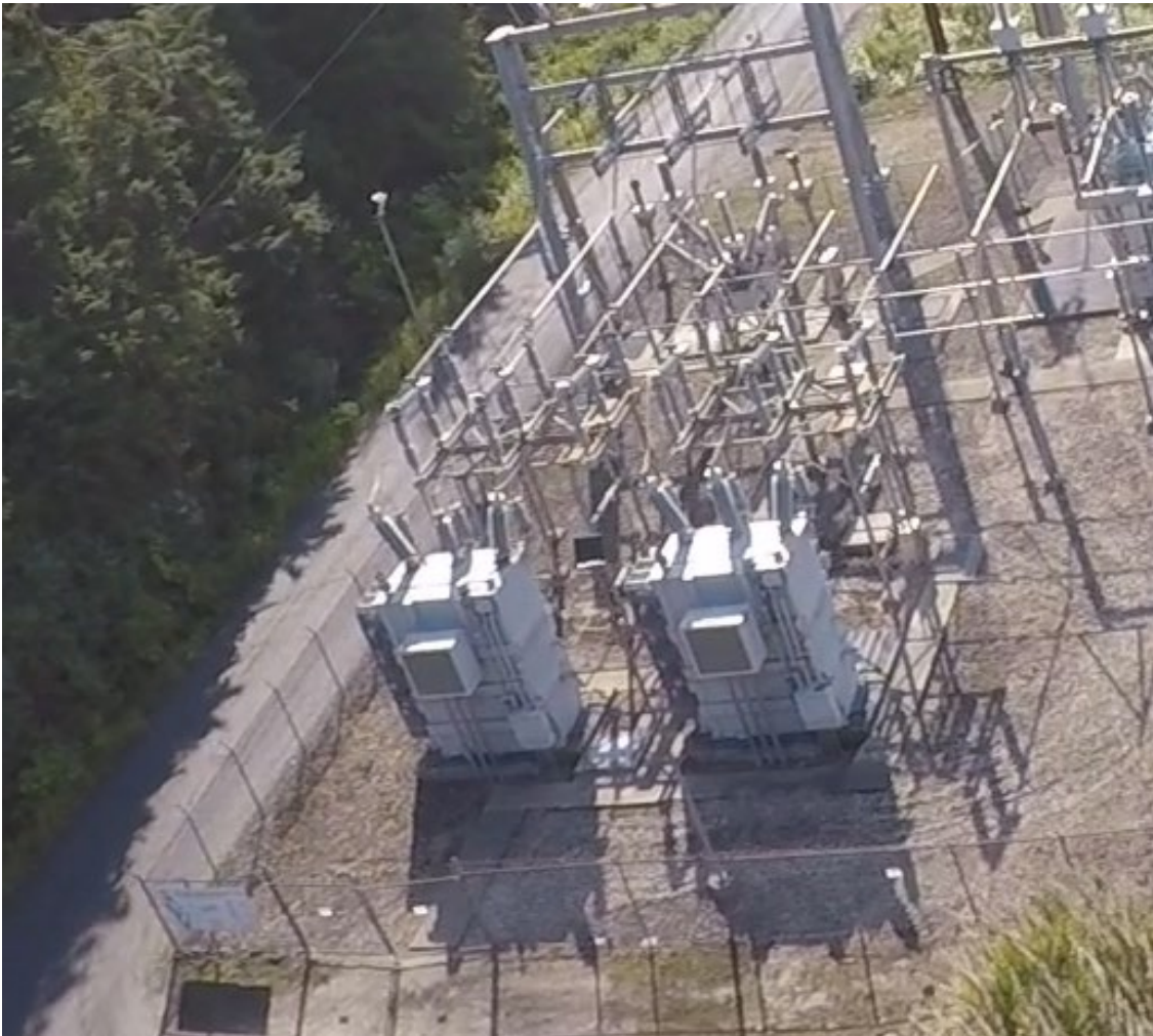
Photo 3-7 Switchyard showing space for installation of third transformer.
