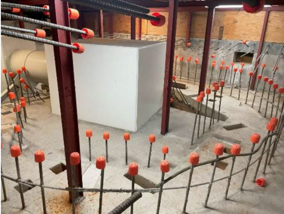
Photo 3-3 Penstock and concrete thrust box in empty bay for the third unit.
