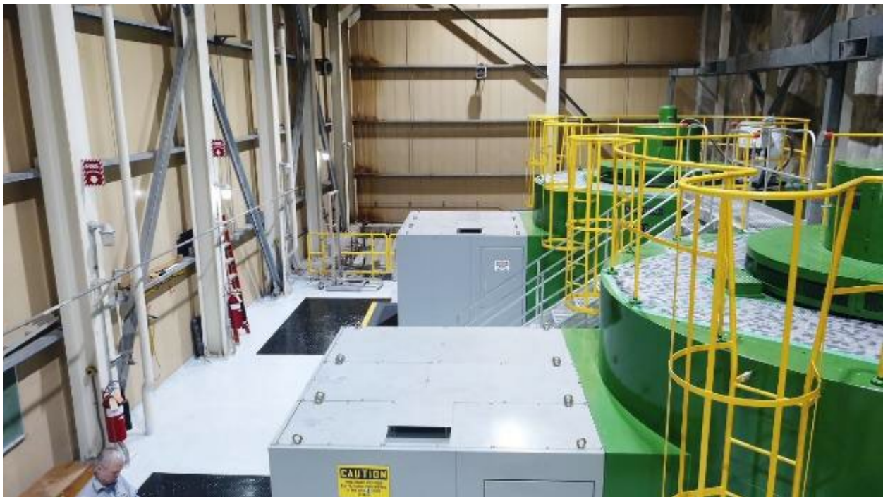
Photo 3-5 Existing turbines in the Tyee Lake powerhouse.
